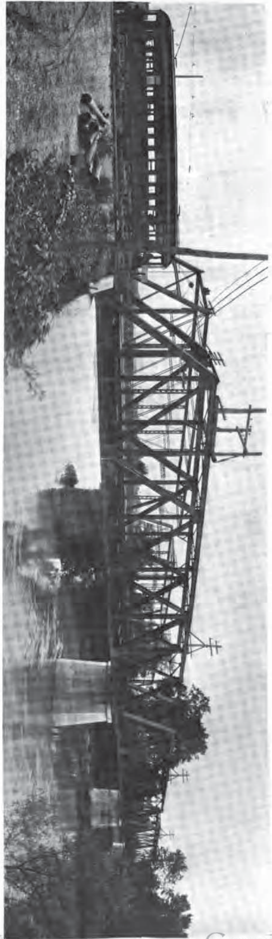
STEEL BRIDGE OVER SCIOTO RIVER AT ENTRANCE TO CHILLICOTHE SCIOTO VALLEY TRACTION COMPANY
